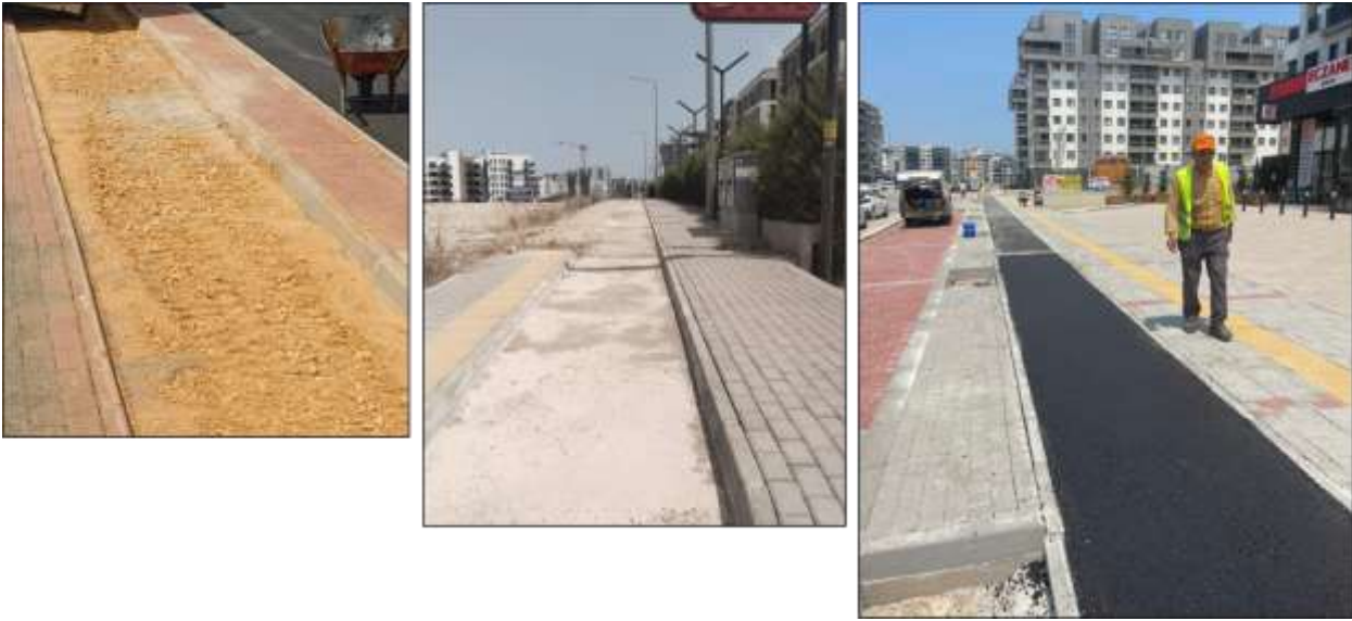
Figure 2: Figure 1: (1) Application of plant mix base as the base for a hot mix asphalt bicycle path. (2) Application of C20/25 concrete as the base for a hot mix asphalt bicycle path. (3) A bicycle path using hot-mix asphalt material.
